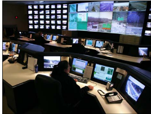
PICTURE 5 – The control room at the VDOT Eastern Region Traffic Operations Center. Photo source: VDOT.
